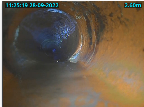
Fig 4.2: Line 4 Joint Displacement and Cracking
