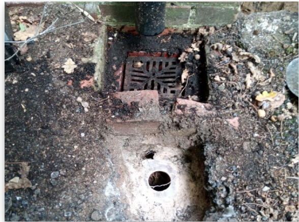
Fig 5.2: RWG2 Break in point
