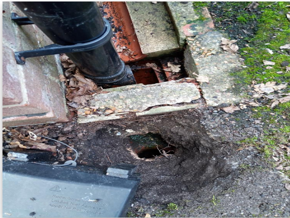
Fig 5.1: RWG1 Break in point
