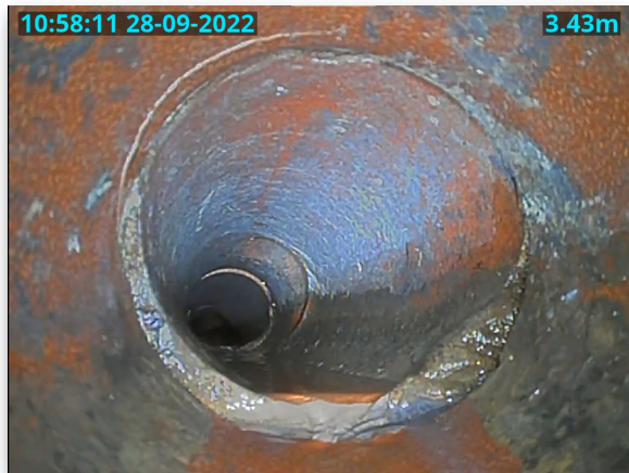
Fig 4.1: Line 3 Joint Displacements and Cracking
