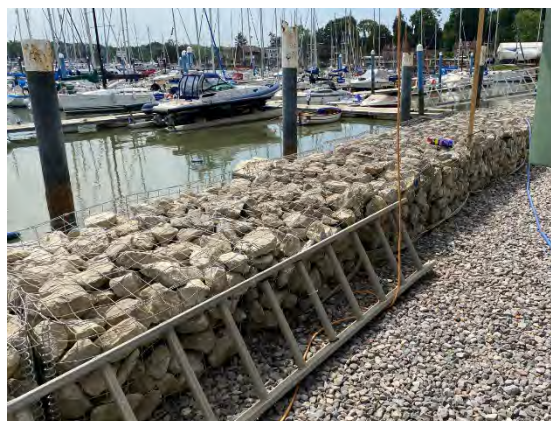
Photo 6: Gabion Wall located along the central southern boundary. Note: these are not flood defences, they were installed to slow erosion
