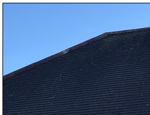
Figure 6 – missing mortar under ridge and hip tiles on main roof
