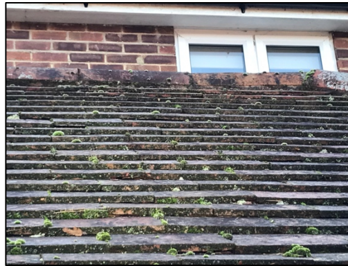
Figure 10 – lifted roof tiles on north-eastern roof face
