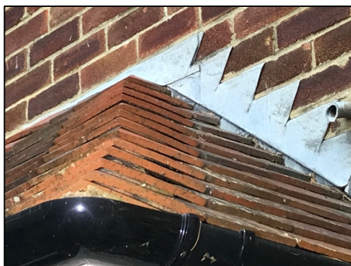
Figure 5 – lifted hip tiles on porch
