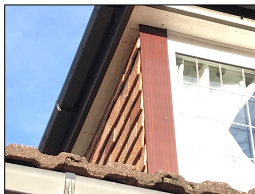
Figure 6 – gaps under hanging tile on dormer windows
