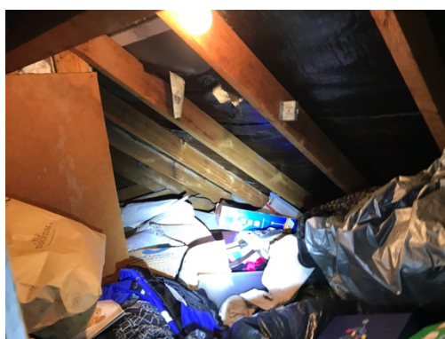
Figure 7 – tears in bitumen lining and hanging folds
