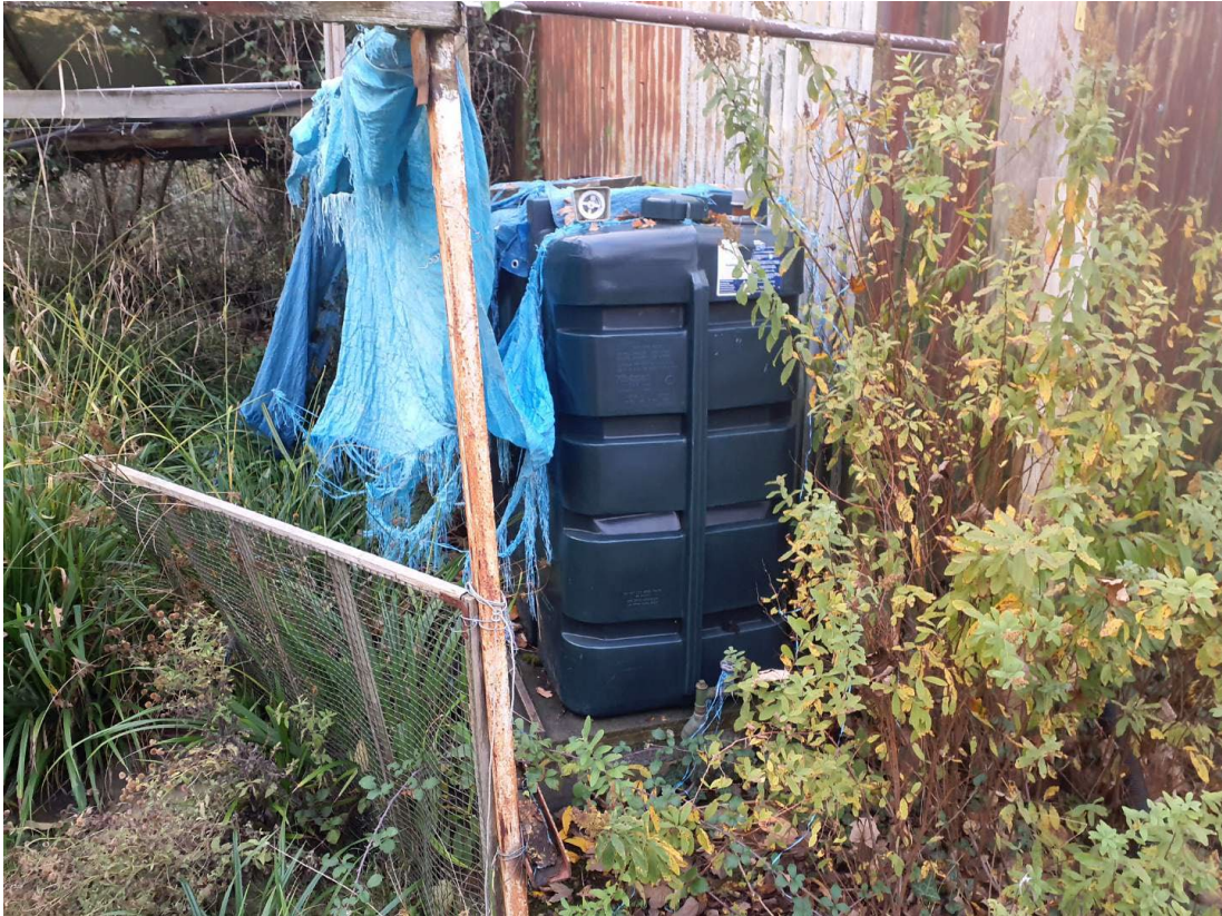
Plate 25: Oil tank behind the western shed. Strong fuel smell.
