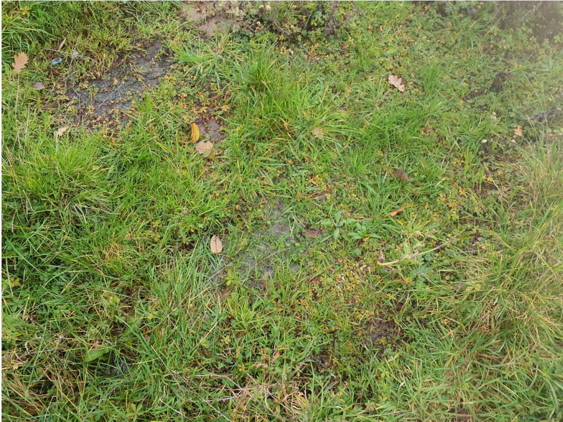
Plate 23: Evidence of high water table in the centre of the site.
