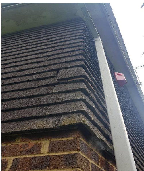
Picture 3: Showing the gaps on the hanging tiles on the north western end of the house
