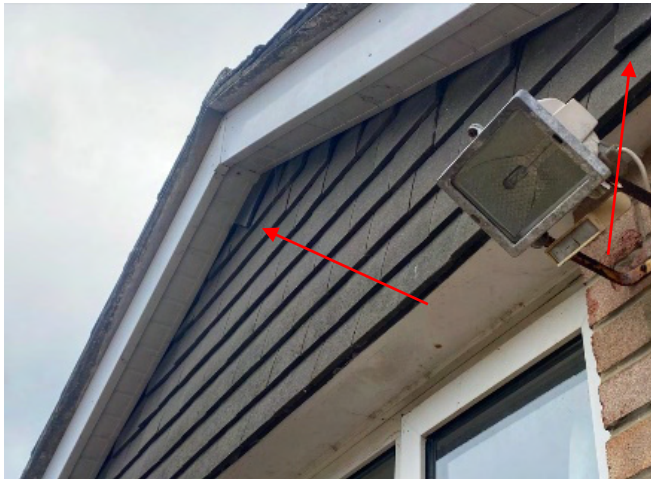
Figure 12. Gaps under hanging tiles.
