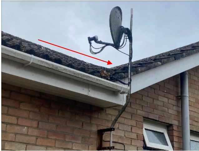
Figure 11. Gaps under the roof tiles.
