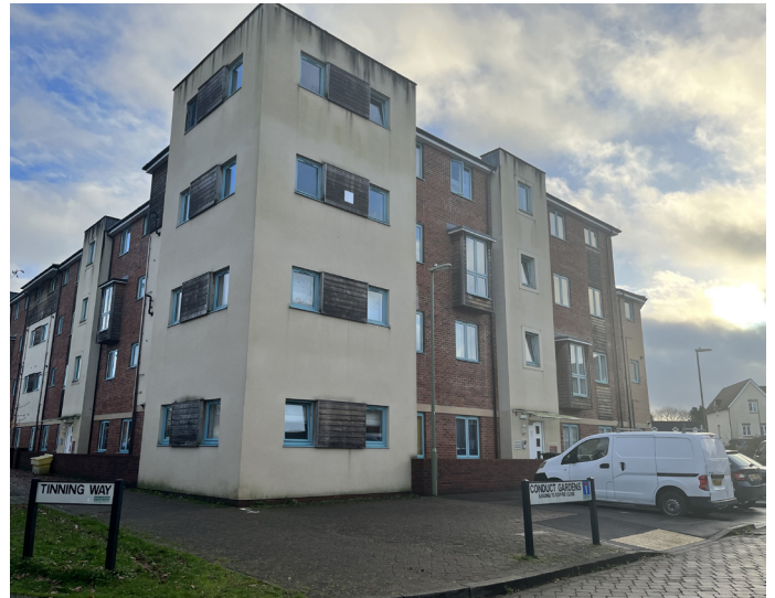
Mix of render and brick facade with panels of timber cladding - hasn't weathered well
