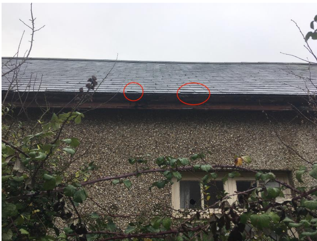
Figure 3: Slate tile roof with potential gaps for bats.
