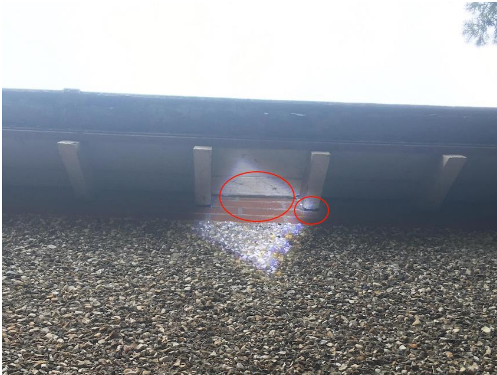
Figure 5: Gap under soffit, to left above, and where rafters protrude through the external wall, to the right above; these were present around the building at different points
