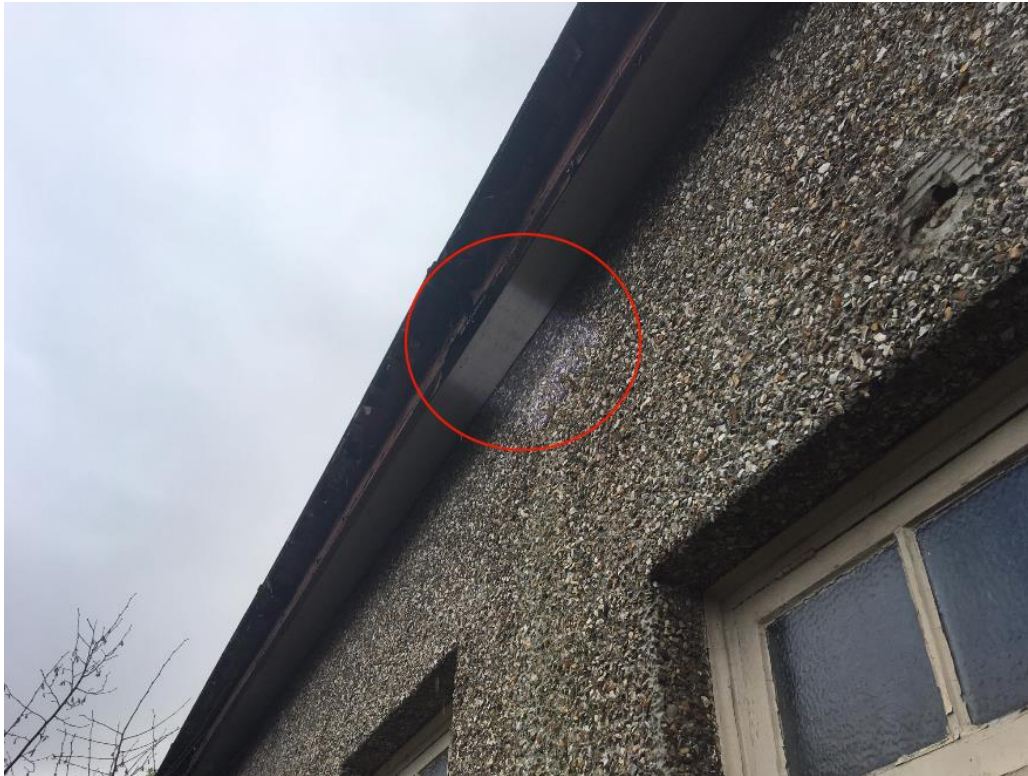
Figure 4: Gap where soffit meets the external wall; this was present around the building at different locations
