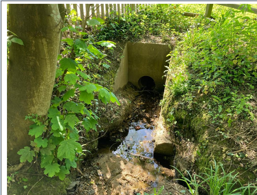
Image 3: downstream gully requiring trash screen
