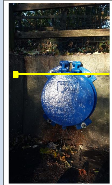
Image 2. Security bar installed here to prevent valve opening more than 90 degrees
