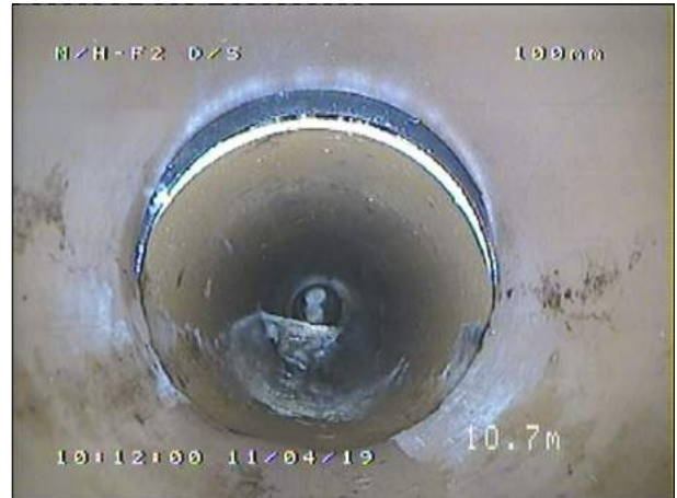
Photo: 1_1_17_A.JPG 10.7m, Sewer material changes
