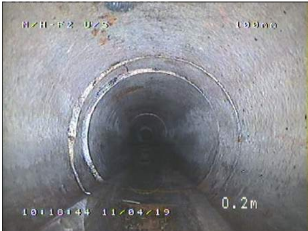
Photo: 3_3_28_A.JPG 0.2m, Fracture, circumferential at joint, from 12 to 12 o'clock, Start
