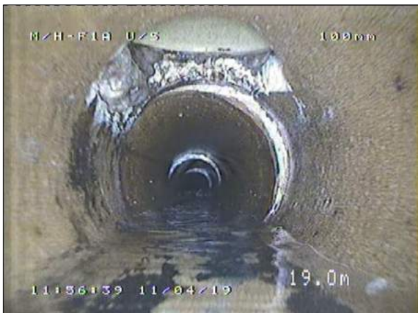
Photo: 12_12_90_A.JPG 19m, Connection defective, at 12 o'clock, 100mm diameter
