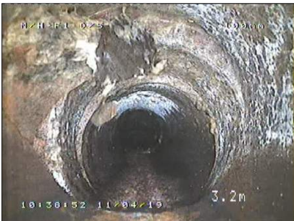
Photo: 9_9_66_A.JPG 3.2m, Broken sewer at joint, from 12 to 12 o'clock
