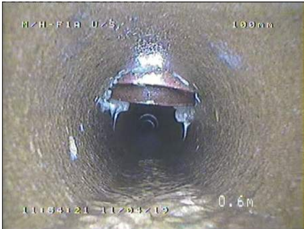
Photo: 12_12_87_A.JPG 0.6m, Connection defective, at 12 o'clock, 100mm diameter, 10mm intruding
