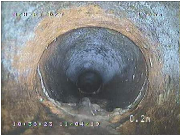
Photo: 9_9_63_A.JPG 0.2m, Fracture, circumferential at joint, from 12 to 12 o'clock, Start
