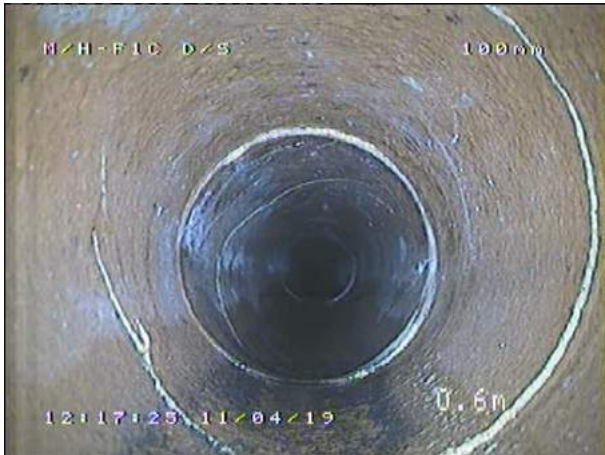
Photo: 17_17_128_A.JPG 0.2m, Fracture, circumferential at joint, from 12 to 12 o'clock, Start
