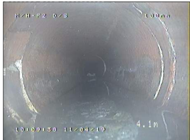
Photo: 1_1_10_A.JPG 4.1m, Broken sewer at joint, from 12 to 12 o'clock
