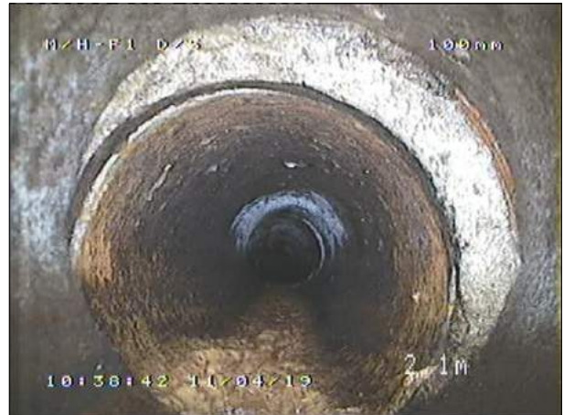
Photo: 9_9_65_A.JPG 2m, Joint displaced, medium (between 1.0 and 1.5 times the pipe wall thickness)
