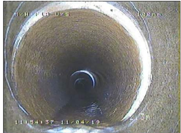
Photo: 12_12_88_A.JPG 2.3m, Fracture, circumferential at joint, from 12 to 12 o'clock, Start
