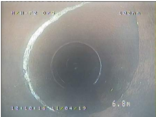
Photo: 1_1_7_A.JPG 2.1m, Fracture, circumferential at joint, from 12 to 12 o'clock, Start
