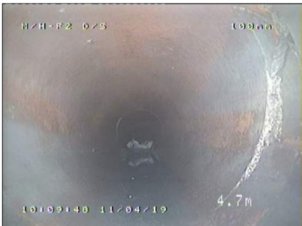
Photo: 1_1_11_A.JPG 4.7m, Broken sewer at joint, from 12 to 12 o'clock
