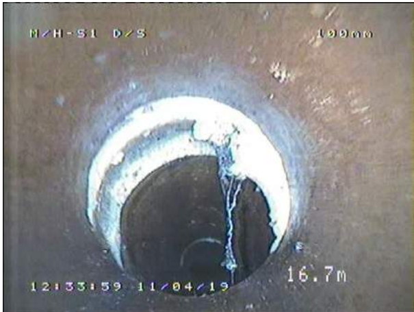
Photo: 18_18_144_A.JPG 15.7m, Line of sewer deviates down, Start
