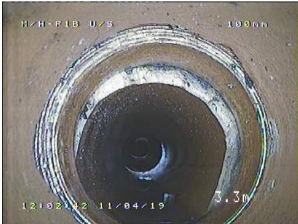
Photo: 13_13_101_A.JPG 3.3m, Broken sewer at joint, from 12 to 12 o'clock
