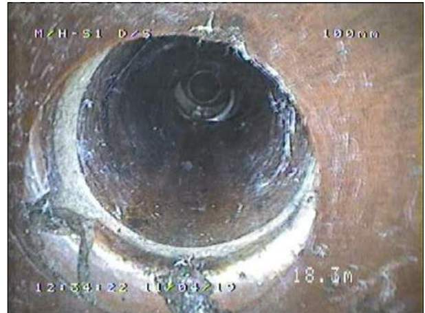
Photo: 18_18_146_A.JPG 18.3m, Line of sewer deviates down, End
