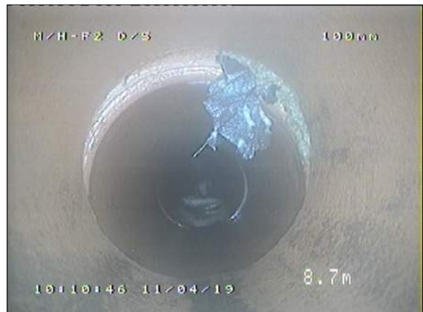
Photo: 1_1_12_A.JPG 8.7m, Joint displaced, medium (between 1.0 and 1.5 times the pipe wall thickness)
