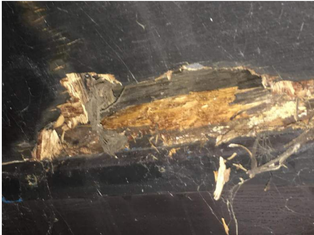
Photograph 15:- Rot affected purlin at back of stage
