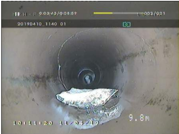
Photo: 1_1_14_A.JPG 9.8m, Fractures, multiple, from 12 to 12 o'clock, Start
