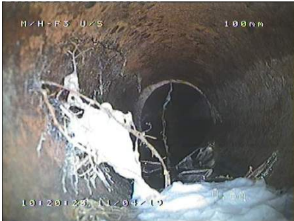
Photo: 4_4_37_A.JPG 0.2m, Roots, fine at joint, Start
