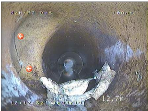
Photo: 1_1_20_A.JPG 12.7m, Junction, defective, at 9 o'clock, 100mm diameter
