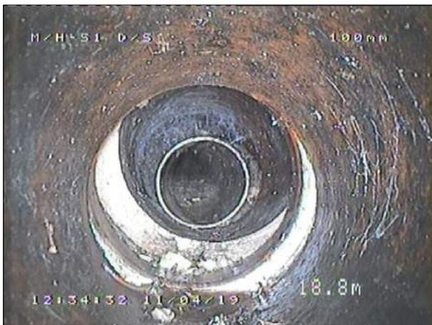
Photo: 18_18_147_A.JPG 18.8m, Joint displaced, large (over 1.5 times the pipe wall thickness)
