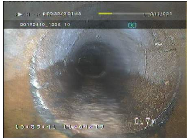
Photo: 11_11_82_A.JPG 0.7m, Fractures, multiple, from 12 to 12 o'clock, Start
