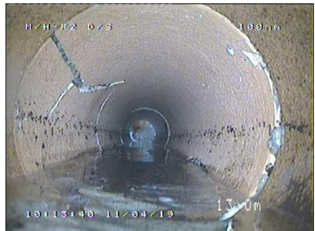
Photo: 1_1_21_A.JPG 13m, Fractures, multiple, from 12 to 12 o'clock
