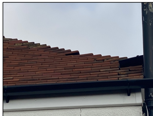
Figure 6 – missing mortar under hip tiles
