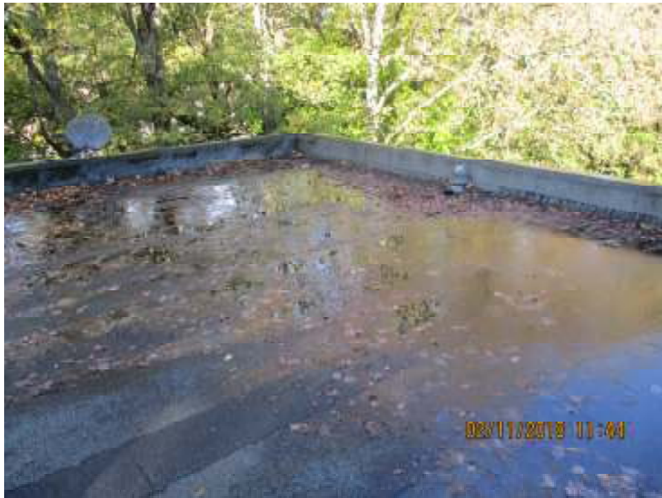
View of the existing roof area showing the ponding
