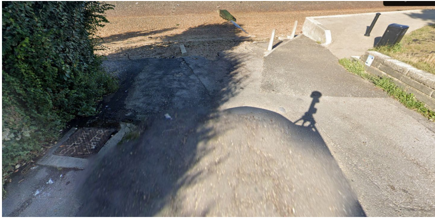
Beach Lane entrance to the beach. Google image August 2020. Very scarred and pot holed surface.
