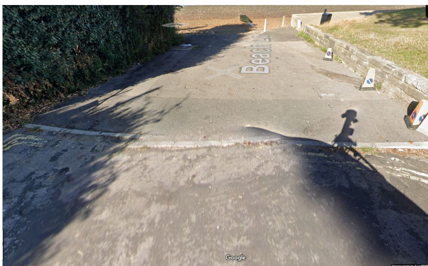
Beach Lane facing the entrance to the beach, close up. Google image August 2020. Very scarred and pot holed surface.
