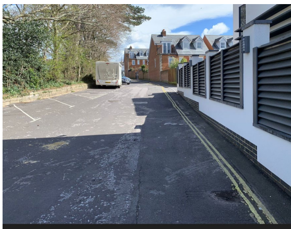
Facing from the beach up Beach Lane. Multiple pot holes and scarred surfaces.
