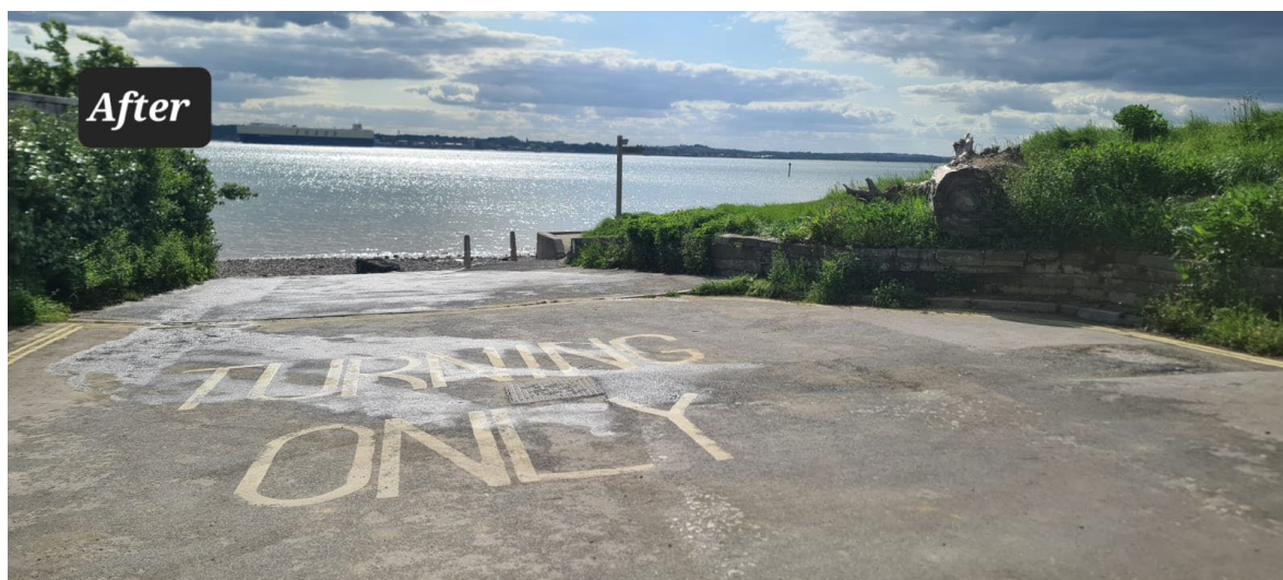
Beach Lane facing the entrance to the beach. Very scarred and pot holed surface as before.
