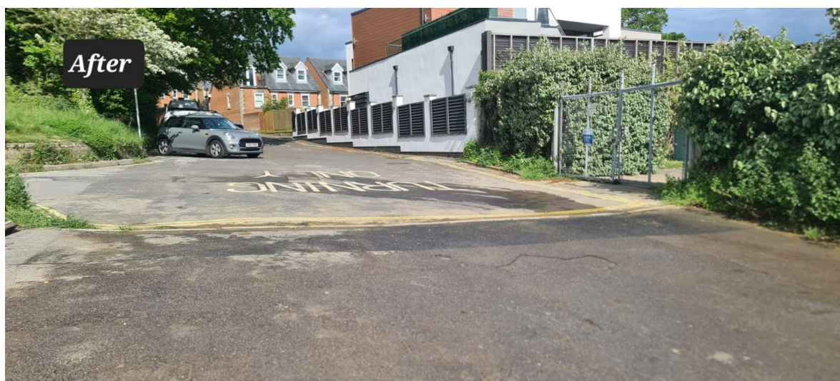
Facing from the beach up Beach Lane. Multiple pot holes and scarred surfaces as before.
