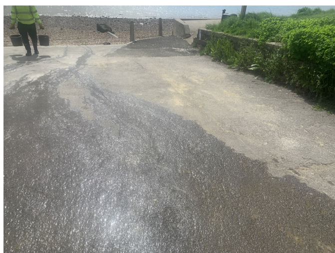
Beach Lane facing the entrance to the beach. Very scarred and pot holed surface as before.
