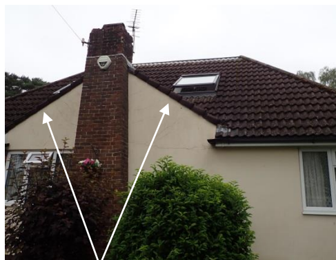
Gaps beneath overhanging edge tiles
