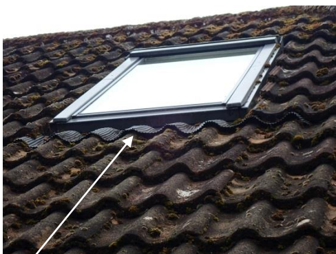
Gaps beneath flashing
