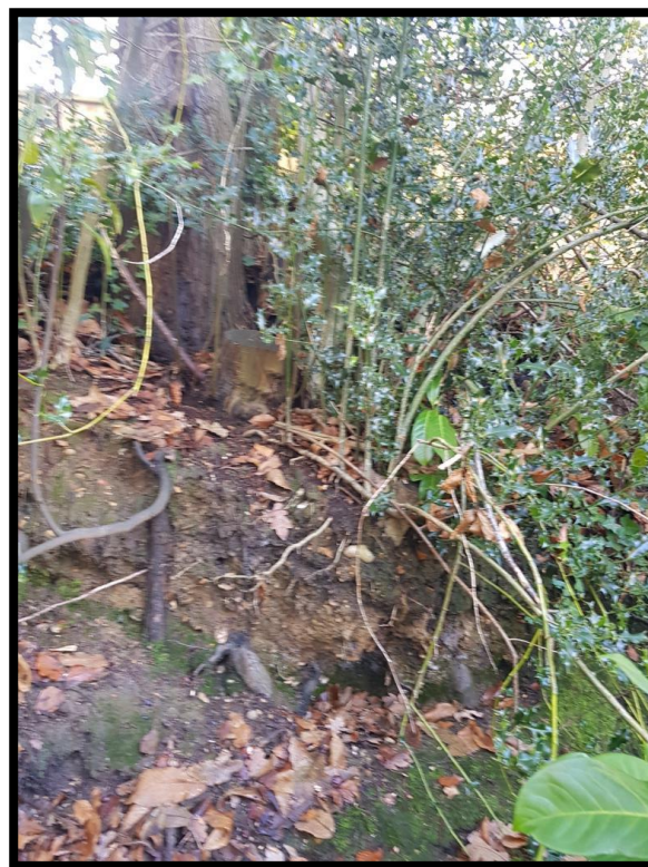
Plate 2: Bank erosion and exposed roots.
