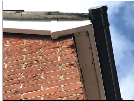
Figure 6 – lifted soffits at back corner section.
