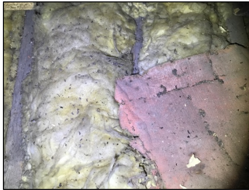
Figure 7 – concentration of long-eared bat type droppings under the front hip in the south-west corner in the roof void.
