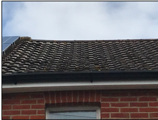
Figure 5 – missing mortar under front ridge tile.
