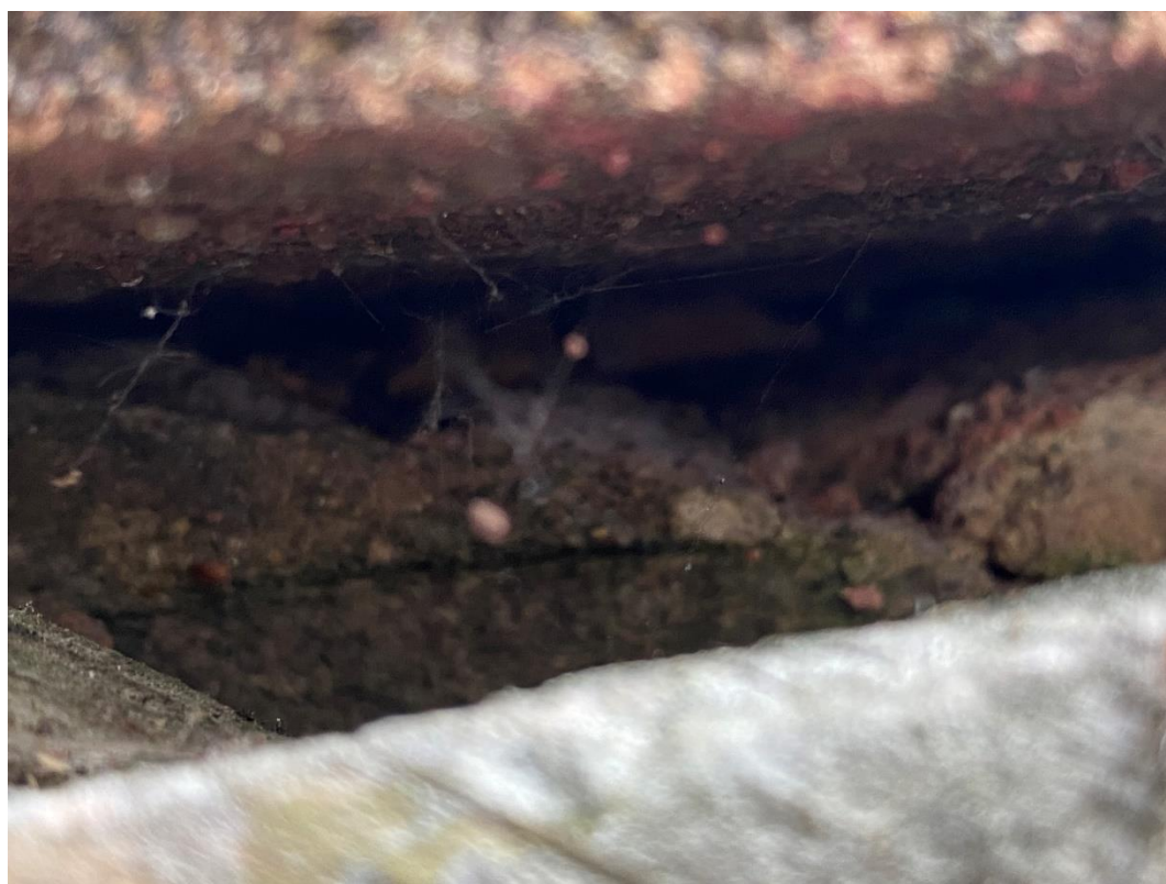
Figure 5. Detail of opening at southwest corner adjacent to gutter: The space beneath is a shallow, closed off opening 40mm deep.
