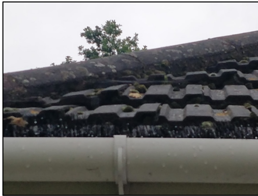
Figure 7 – lifted concrete tiles
