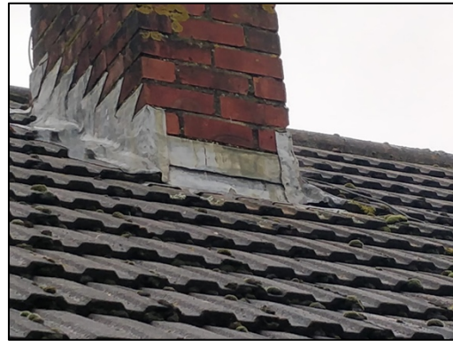
Figure 8 – sections of lifted lead flashing around chimney
