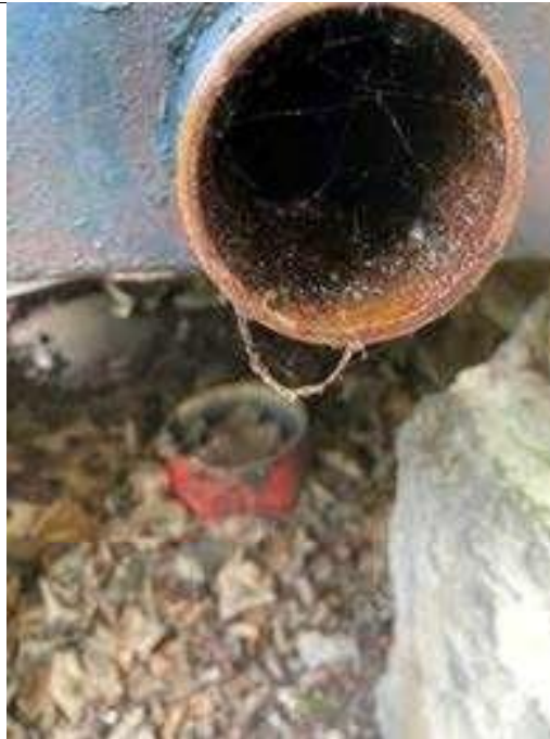
Photograph 6- Tar Substance within pipe of rusted green tank on northern boundary. Facing west.
