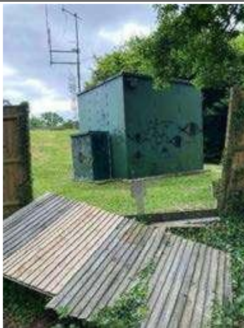
Photograph 7- Electrical substation on the southern boundary of the site, within neighbouring property. Facing South.
