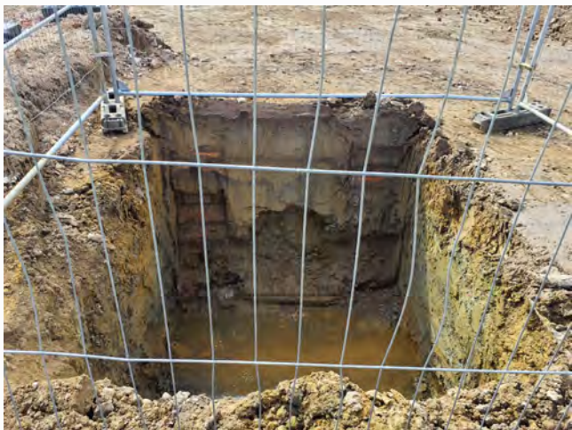
Description Area C tank
