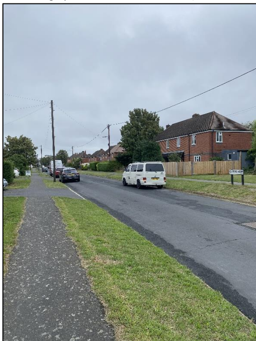
Photograph 4: Queens View Footways
