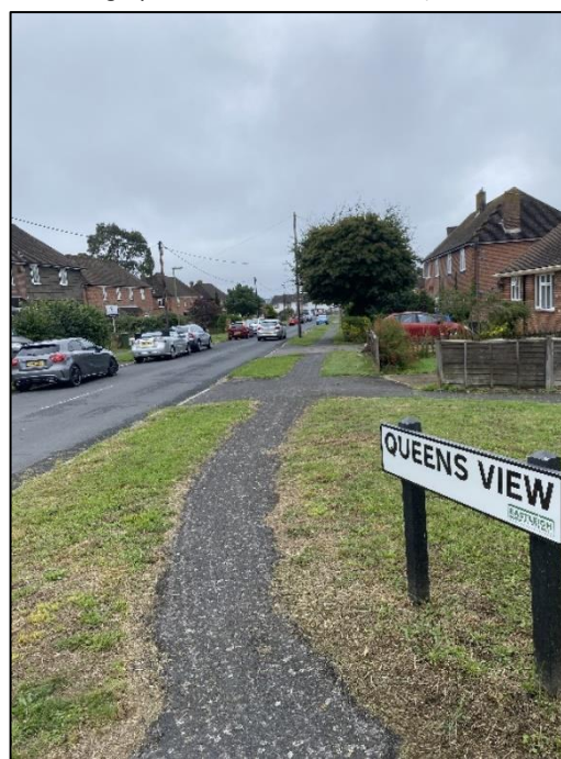
Photograph 5: Queens View Footways
