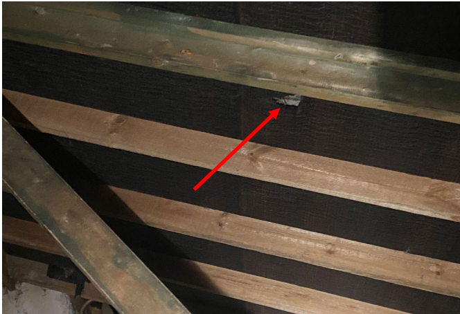
Figure 21. Gaps in the bitumen lining of the loft space of 32 Queens View (taken June 2022).
