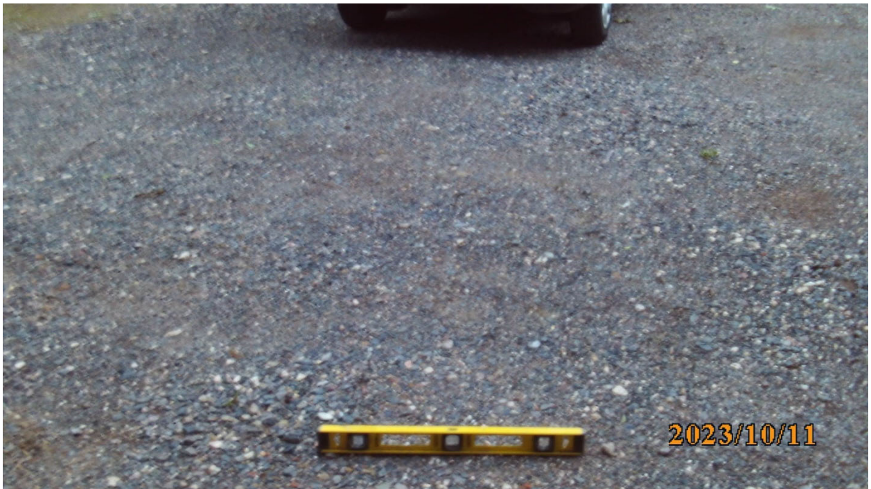
Pavement fall to the north west
