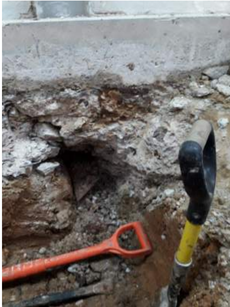
Photo 5: Image of TP04. Note the steel penetrating through the concrete and protruding out of the base of the concrete.
