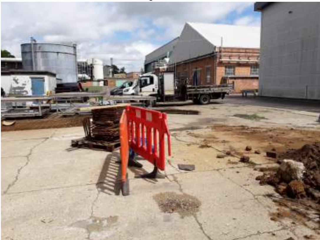
Photo 8: Image of stored equipment.
