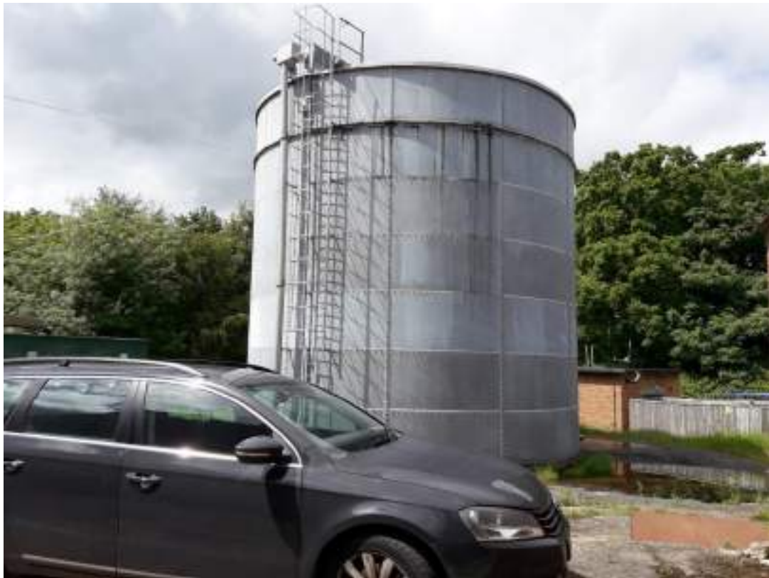
Photo 5: Image of tank containing water for sprinkler tank and associated buildings located north of Site.
