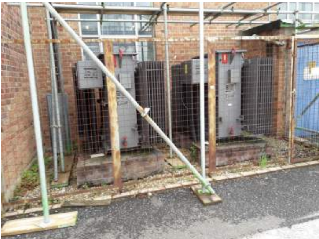
Photo 6: Image of electricity sub-station 15m west of the Site.
