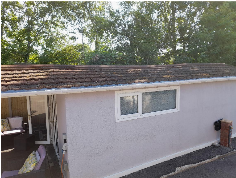
Existing amenity building to be replaced. It has a leaking and sloping roof.
