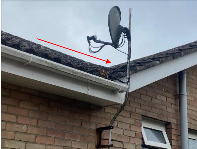
Figure 11. Gaps under the roof tiles.
