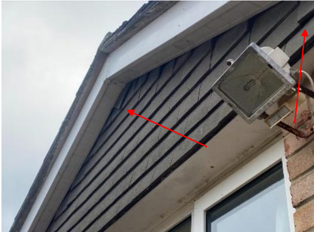
Figure 12. Gaps under hanging tiles.
