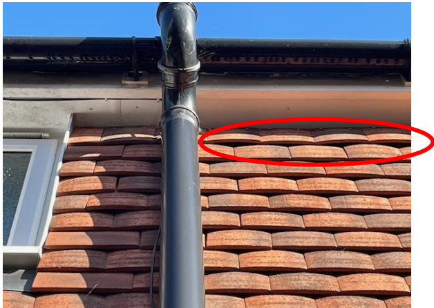
Photo 4: Gaps at hanging tiles.
