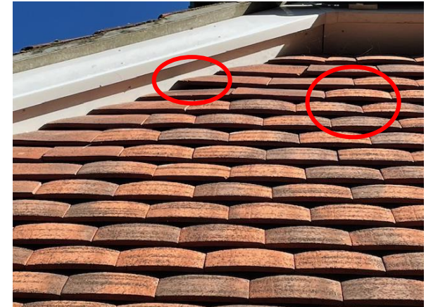
Photo 3: Gaps at hanging tiles.
