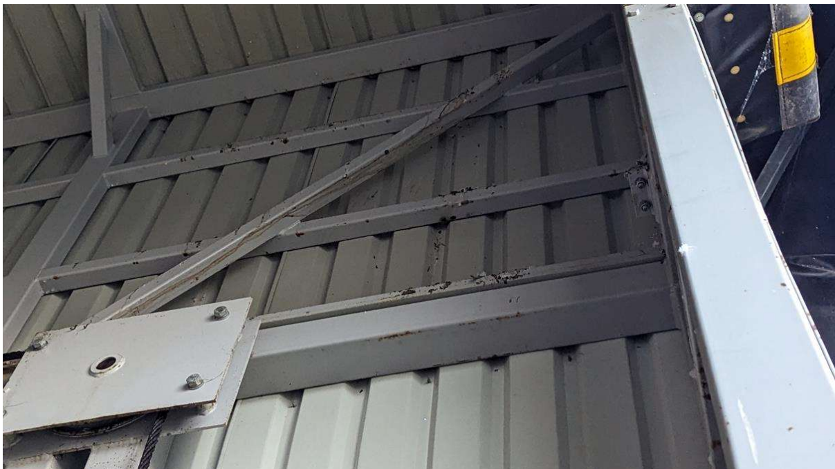
Photo 3 Evidence of birds perching inside the loading bays.
