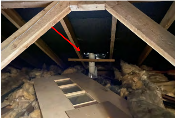
Figure 17. Gaps in the bitumen felt around a pipe (taken June 2022).
