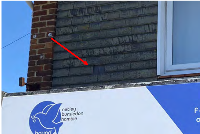
Figure 15. Broken tile on the front (southwestern) face of the building (taken June 2022).
