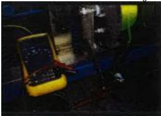
Figure 21 - Earthing (Bonding) Cable
