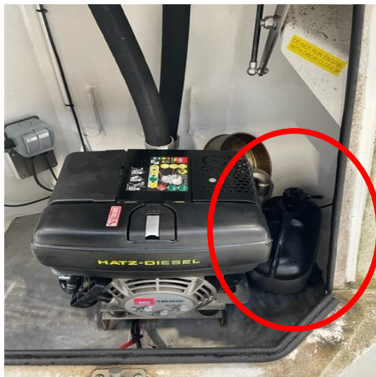
Figure 1 - Incorrectly Stored Fuel Container
