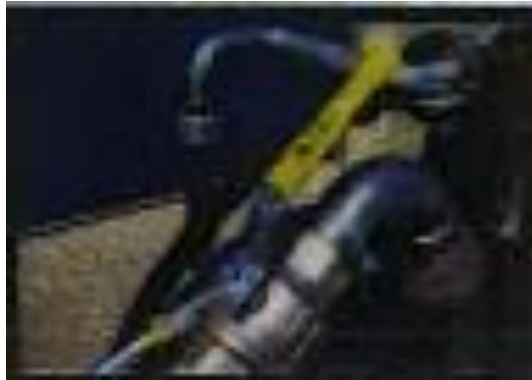
Figure 24 - OPEN Suction Pipe Valve
