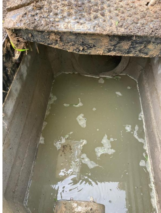
Figure 1.7b: S15 Control Manhole
