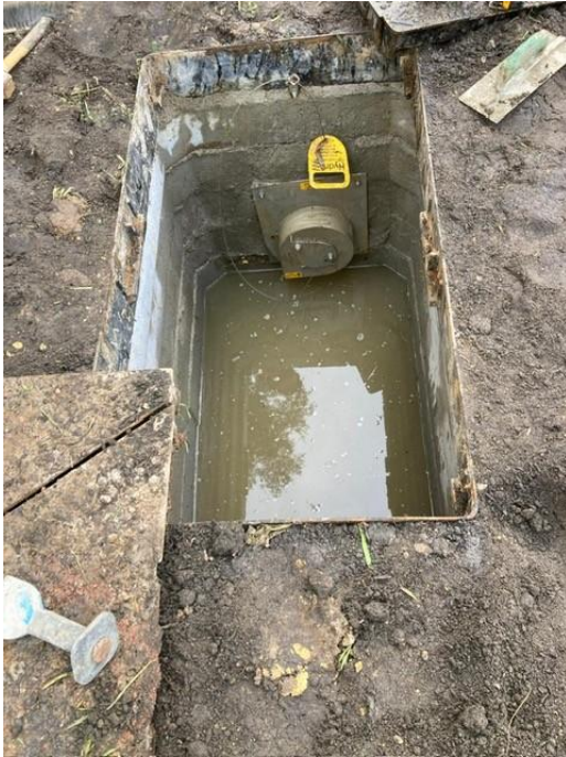
Figure 1.7a: S15 Control Manhole
