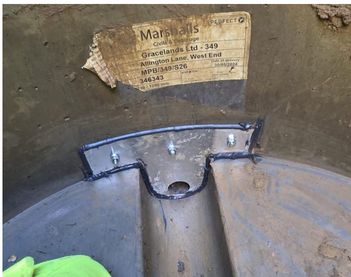
Figure 1.5: 50mm Orifice plate installation
