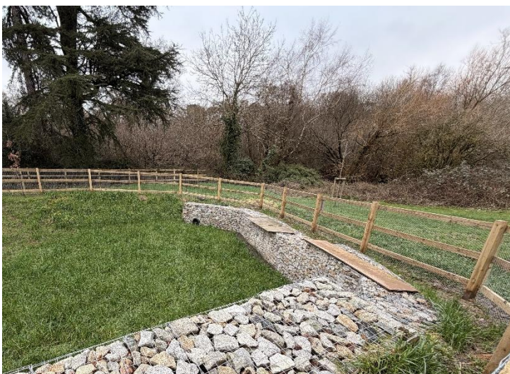
Figure 1.2: Outlet to new flow control chamber
