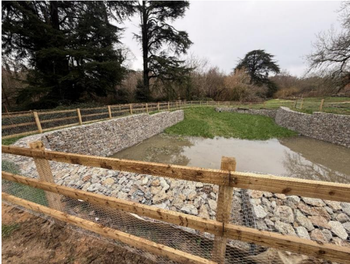
Figure 1.1: SuDS feature, view to outfall from northern gabion structure.
