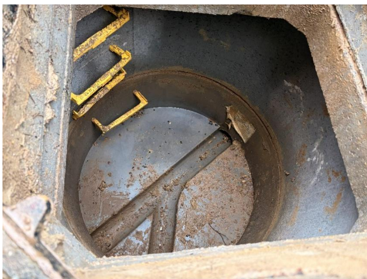
Figure 1.4: S26 Control manhole
