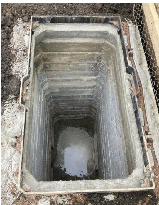
Figure 1.6: S14 Control Manhole
