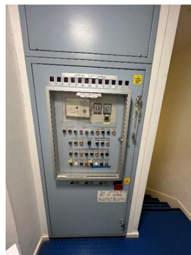
Fig 14. Original control panel within designated escape route.
