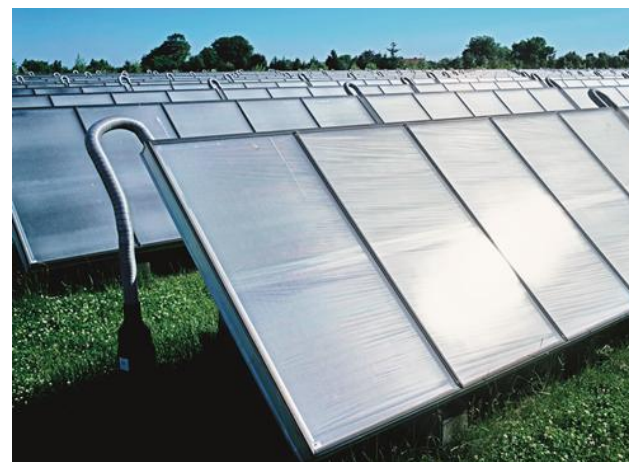
Figure 2.2 – Solar Collector Array
