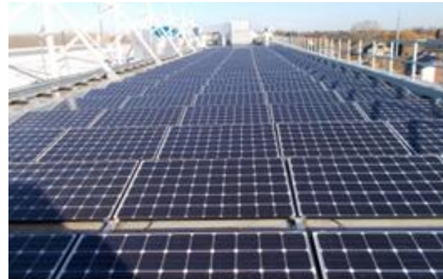
Figure 2.1 – Photovoltaic Panel Array
