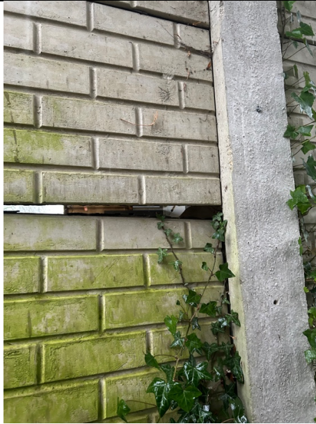
Gaps in wall at rear of building
