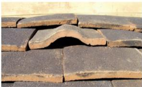
Raised roof tiles © Darwin Ecology
