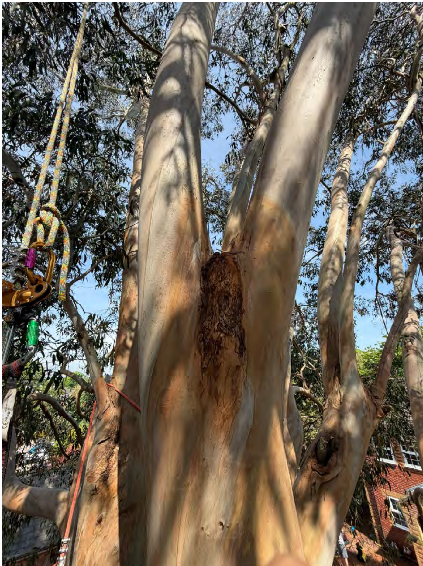
Image 16: Close-range view of a specific compression union at approximately 8m AGL. The extended, elongated dark-stained zone between two co-dominant stems is clearly visible. The angle of the branch bark ridge and the presence of this staining zone, extending vertically downward from the union, are diagnostic of a compression union in which bark has been occluded between the stems under prolonged compressive loading.
