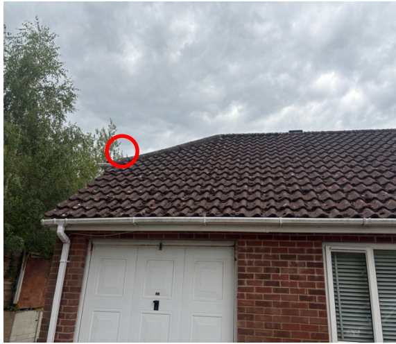
Photograph 1. A small gap in the tiles on the western elevation (red circle).
