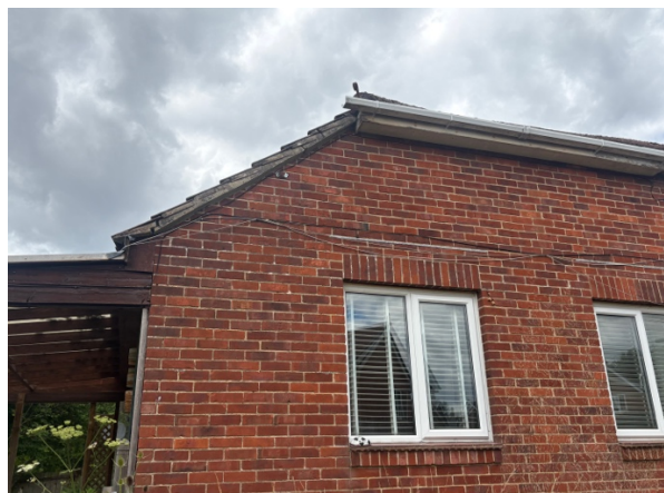
Photograph 6. A small gap in the mortar on the leading edge of the eastern elevation.
