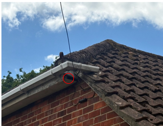
Photograph 5. A small gap in the soffit box on the eastern elevation.
