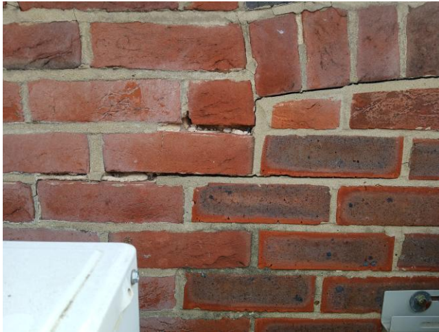
Photo 5: Superficial missing mortar on the western elevation.
