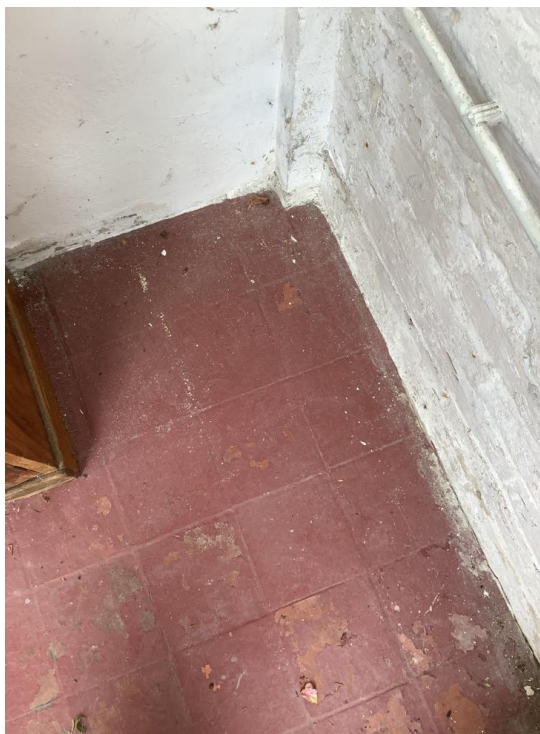
Looking down at the portico's floor – no gapping where the structure meets the front wall of the main building or to the side privacy brick wall thereby confirming that the dropping of the floor slab is historic (taken 05.06.26)
