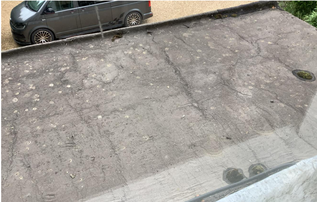
Perished felting roof to canopy over portico – roof covering needs replacing (taken 05.06.26)
