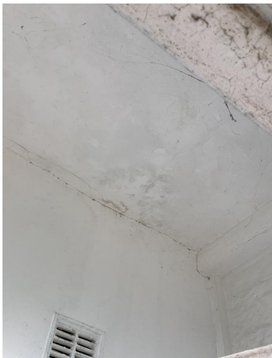
Water staining to the underside of the ceiling – roof finish is starting to perish suggesting it is at the end of its useful life and as such, needs replacement (taken 05.06.26)
