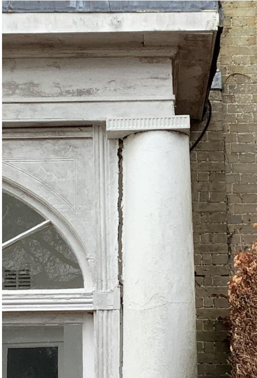
Figures 13: Top of right hand column showing movement Externally
