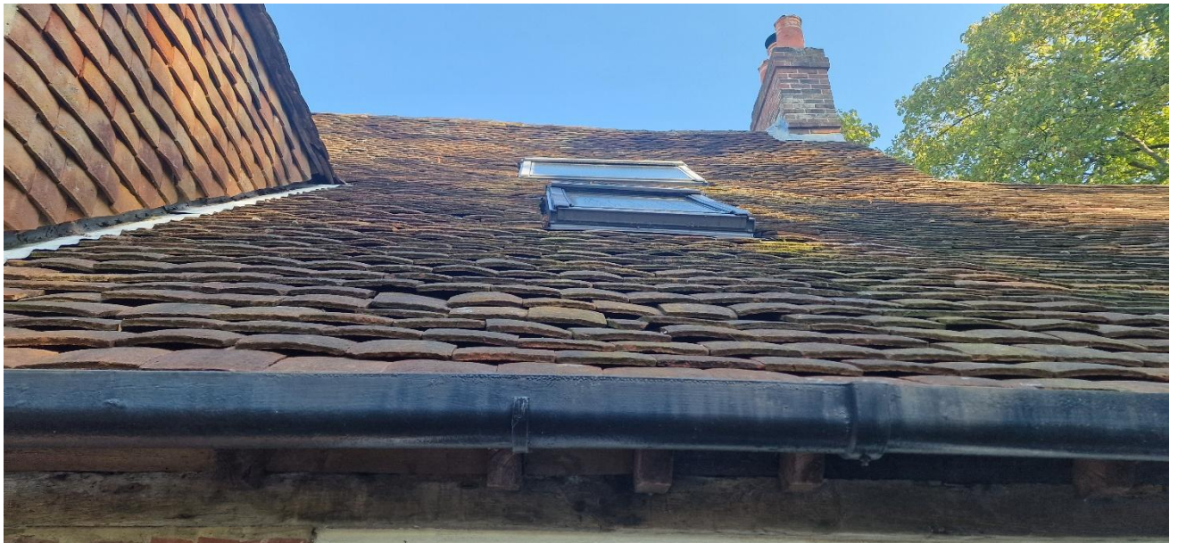
Picture 2: Showing profiles in the tiles that could allow bats to enter
