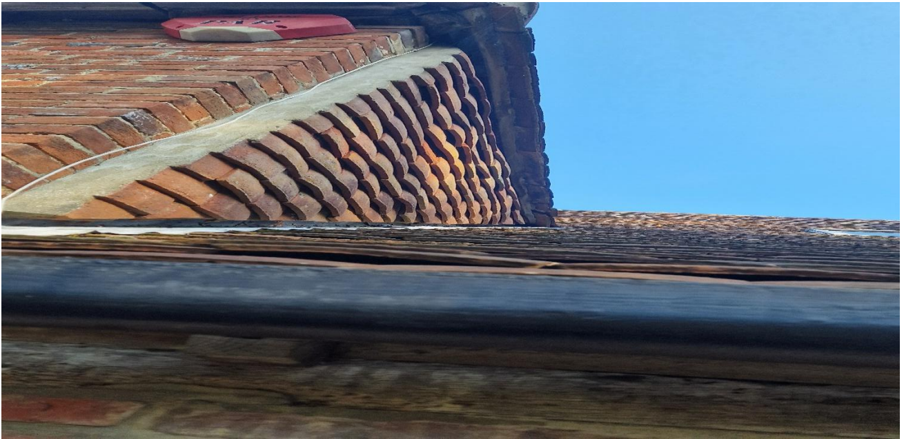
Picture 3: Showing existing hanging tiles and gaps within the tile bed.
