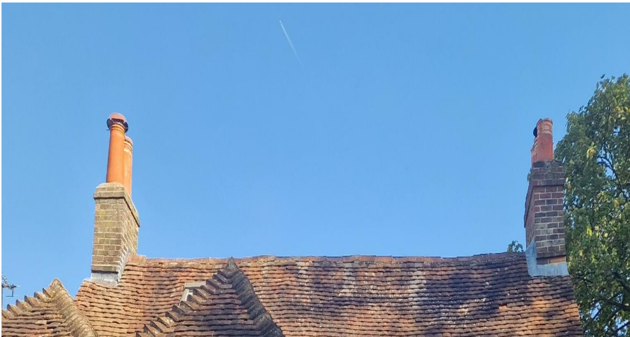
Picture 6: Showing ridge of the main roof and the gaps in the bedding
