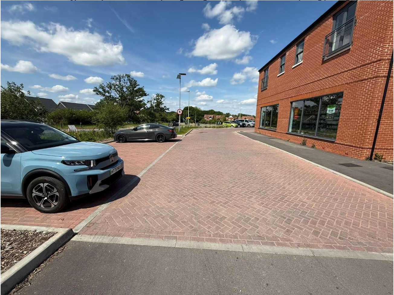
Photo 5: View onto typical impermeable block paving falling towards permeable block paving parking spaces.
