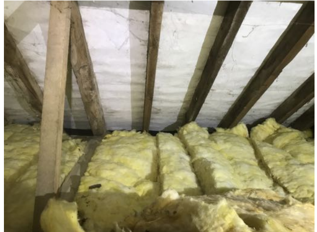
Image 24: Eaves of the northern area of the void. The polythene layer is visible at the base of the eaves
