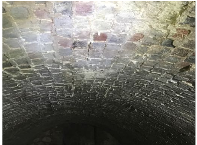
Image 26: Areas of missing mortar within the cellar
