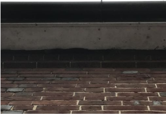
Image 17: Damaged soffit box on eastern elevation of B1
