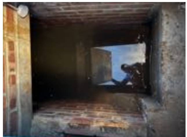
Image 28: Internal entrance to the cellar. The cellar is flooded to ceiling level at the time of the photo - dated 9th January 2025.
