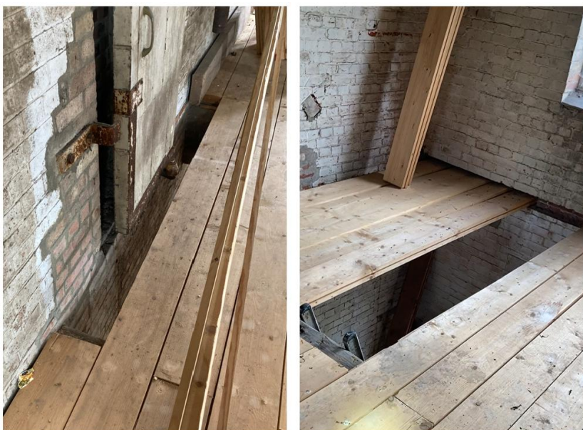
Figure 8. Images of the holes through to the floor below.
