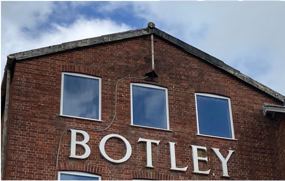
Figure 4. Image showing a wide gap beneath the fascia on the front elevation
