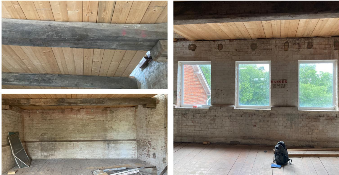
Figure 9. Images of the holes through to the floor below
