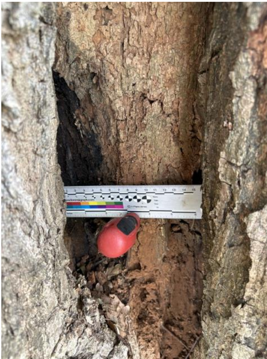
SAL5 Cavity at base of T1.
