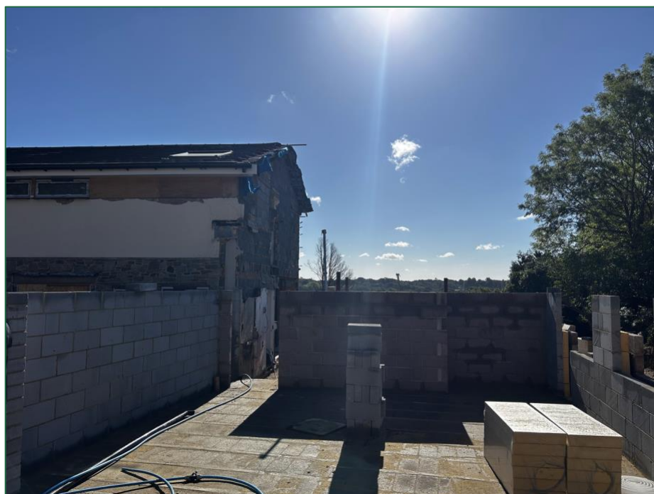
Photograph 5 – Garage (B2), unroofed blockwork shell and junction with the main dwelling, showing the absence of any roof covering or void.
