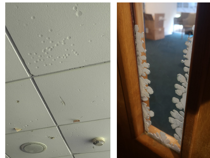
Figure 3.13 Several fire doors in the Rod Bransgrove Pavilion show condensation issues that might compromise its performance
