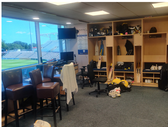
Figure 3.11 Players changing rooms which are too small. The lockers show evident signs of deterioration
