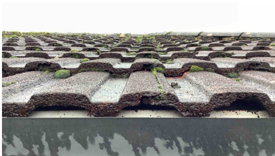
Photograph 3. Roof of B1 showing areas of missing mortar under roof tiles.
