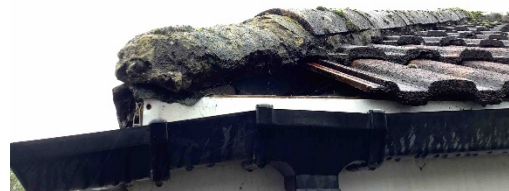
Photograph 4. Roof of B1 showing missing tile and gaps between mortar and tiles.
